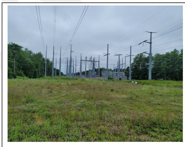
Figure 7 – North of Site – View to the West of Eversource Substation (view as of 13/Jul/2021)
