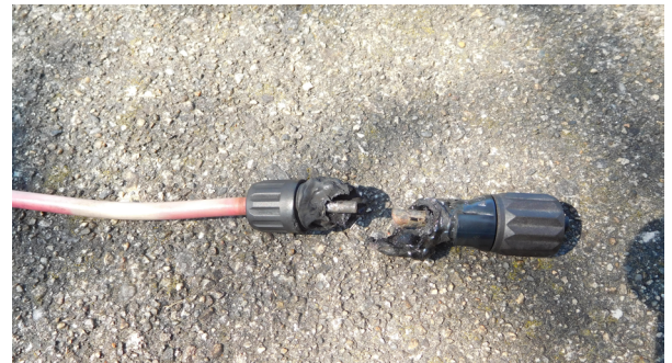
Figure 3. Connectors may fit together but might not make a good electrical connection.
