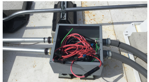
Figure 4. Wires can pull out of connector when poorly made field connection is installed
